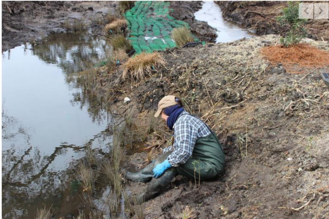
Vicky Smith, a mosquito control and stormwater inspector, installs rushes in the recently constructed wetland in Murrells Inlet.
